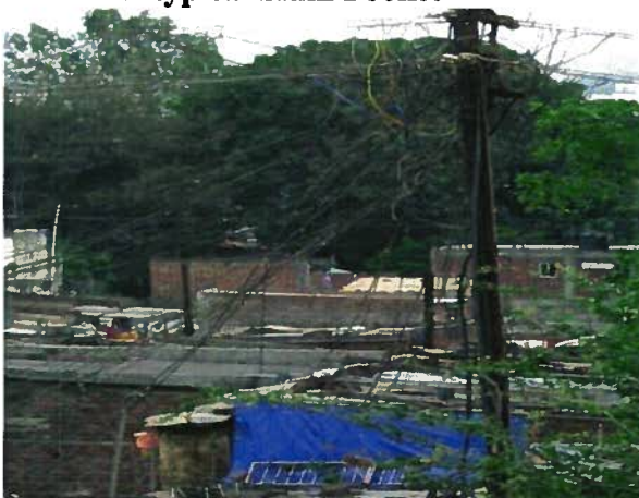
Live Electric Wires Hanging Dangerously over the Hutments
