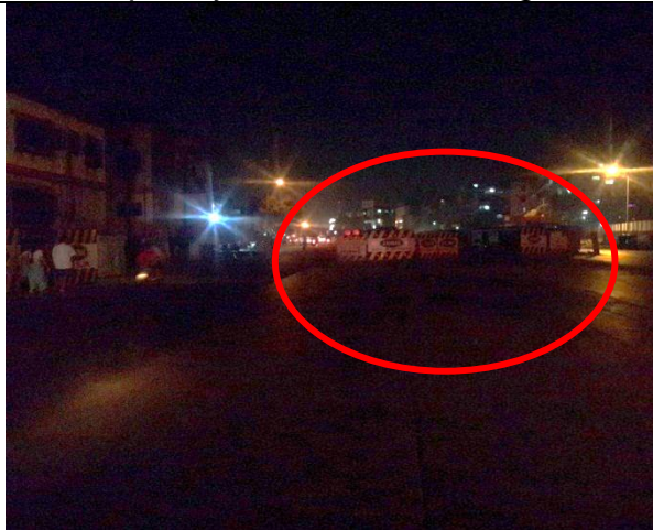
Chainage 3/100 RHS side 18.472608, 73.856325: Sudden reduction in the carriageway by barricading without adequate warning needs to be rectified by erecting advanced warning signs at the start of construction area of Dhankawadi flyover. The reflectors/ reflective material on the barricades are not enough to clearly mark the restricted carriageway width. Traffic blinkers and directional indicators need to be installed to guide vehicles.
