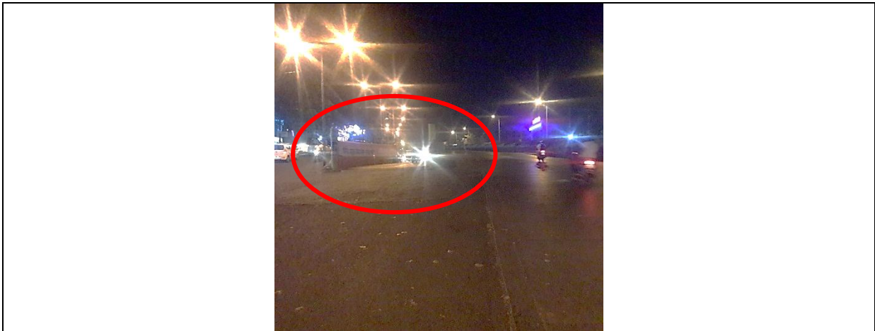
Chainage 1/350 RHS side 18.460213, 73.858213: Entrance to the vehicular subway to Bharati Vidyapeeth lacks any advance direction signage. The RCC walls at the entrance of the subway lack any hazard marker, retro reflective board etc.
