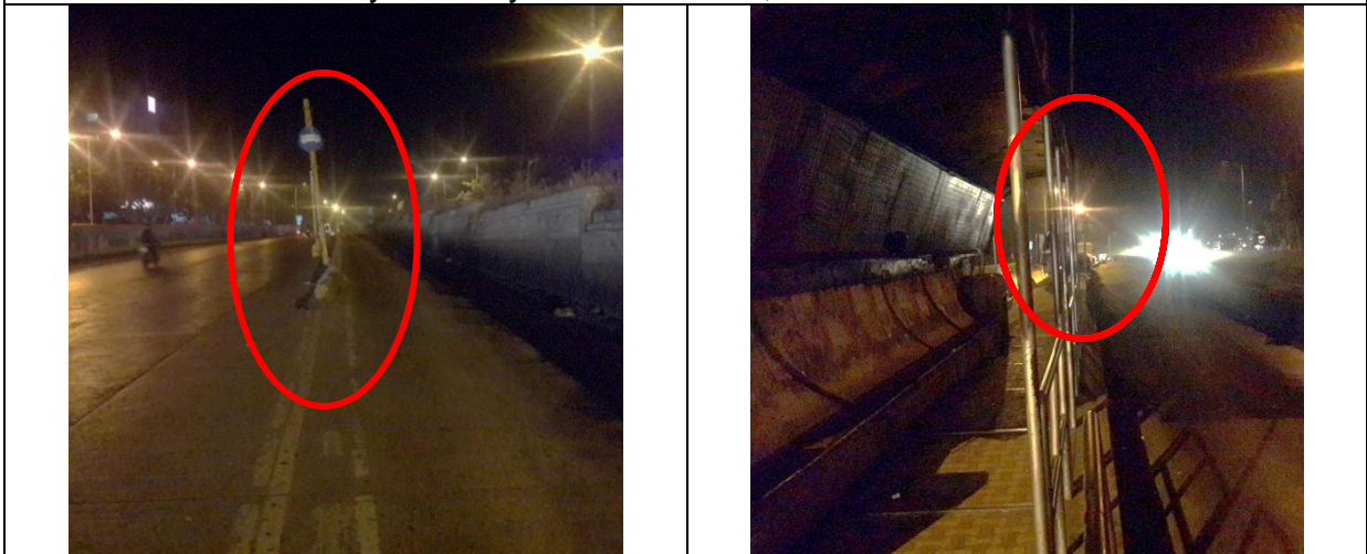
Chainage 1/300 RHS side: The BRTS corridor starting abruptly in front of Bharati Vidyapeeth gate without advanced warning or hazard marker on the kerb / chevron marking etc. Bust stop in front of Bharati Vidyapeeth is without any light arrangement.
