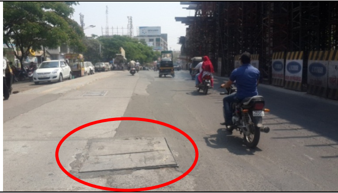
Near Balaji Nagar Junction (Chainage 2/ 550 m RHS side 18.468892, 73.857927) – Protruding frame and RCC chambers of utilities create obstructions in the main carriageway.
