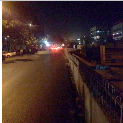
Chainage 3/000 RHS side 18.471570, 73.856947: Exposed reinforcement of ramp wall at the approach to flyover along the main carriageway near Shankar Maharaj
