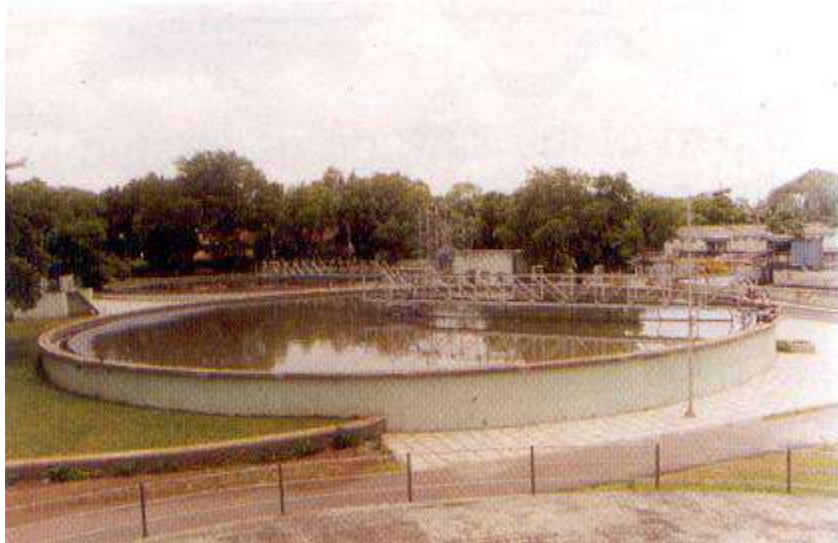
SECONDARY SETTLING TANK AT DR. NAIDU TREATMENT PLANT
